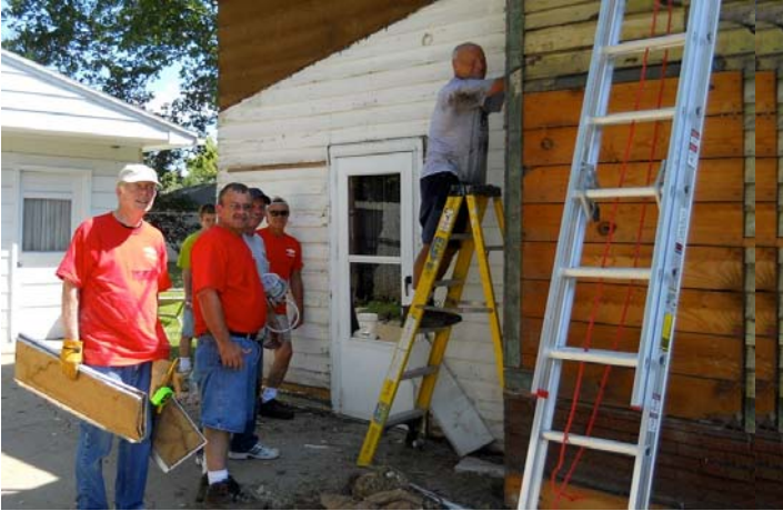
Ss. Peter & Paul members installed siding, windows, doors, steps and insulation. Great job!
