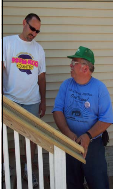
Clay Strait (right) helps Doug Kadolph with a railing on the GM Powertrain house.
